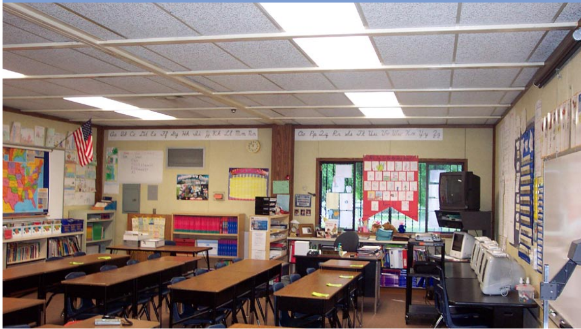
A FUSD portable classroom with a completed lighting upgrade
