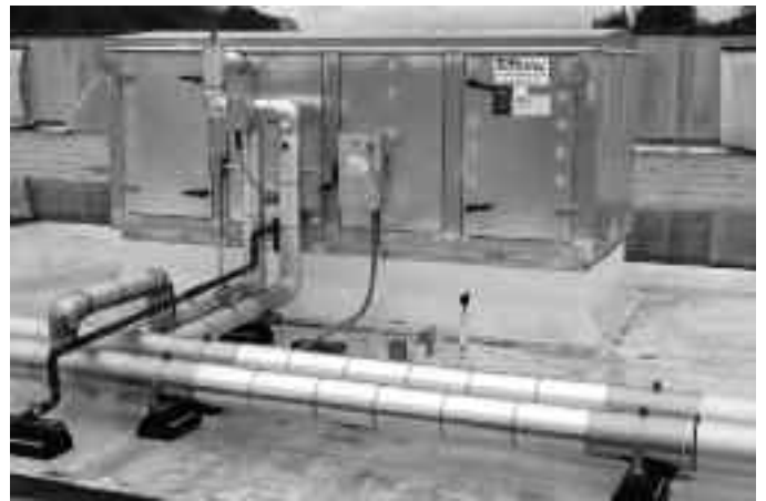
Six air-handlers atop the barrel room and five atop the casegoods warehouse, are key components of the energy-efficient new system.
