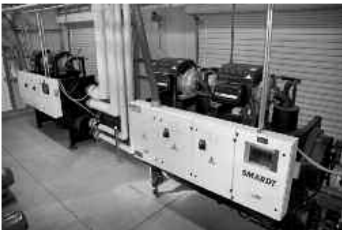
The Smardt chillers are water-cooled and have magnetic bearings, reducing friction, energy use, and maintenance costs.
