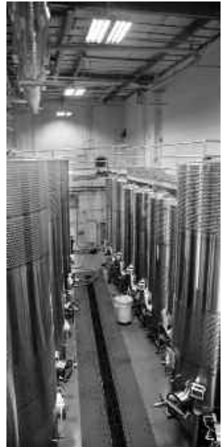
T-8 fluorescent lighting in fermentor rooms, casegoods warehouse, and barrel room reduces energy use by 58,215 kWh per year.
