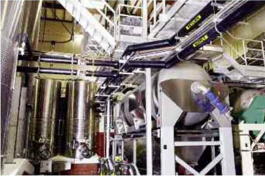
COOL-FIT ABS Plus piping supplies and returns chilled water to fermentation tanks. [Left center, above tanks] Manual COOL-FIT ABS 546 ball valves can isolate supply and return to individual tank aisles.
